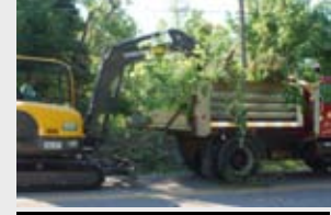
D. Miller and Ivan Clifford clearing ditches of evergreen trees on Hood Road
