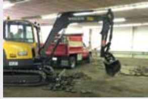
Clearing the wood brick floor from garage of future Police Department at Weymouth Bldg.
